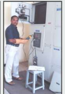
Harmonic Audit at M.V Panel ACB Incoming
